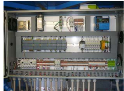
Standard Control Panel with Siemens S7-1200F Safety PLC, automatic circuit breakers, Ethernet Switch, and Honeywell Flame Safeguard.
