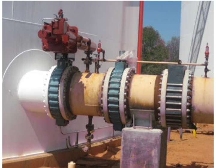
Inlet valves on a tank need to be able to withstand, and close against, high pressures routinely as it stores the various liquids, gases, and produced water.
