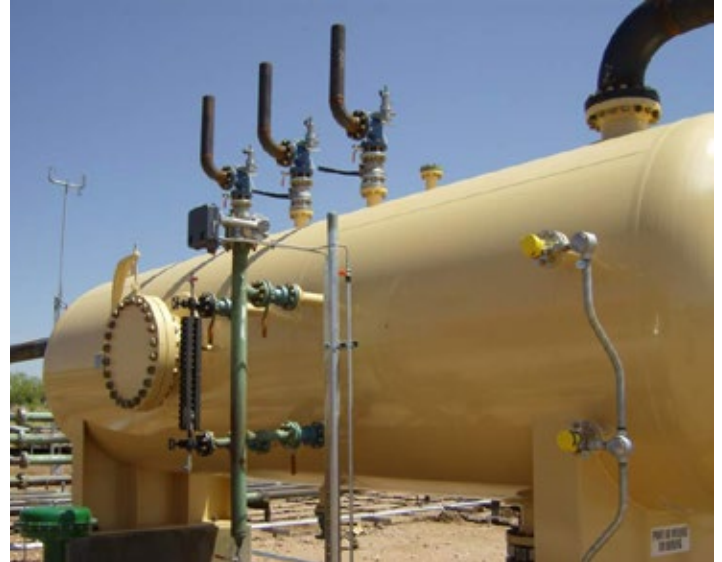
Valves used during separation must be designed to last since the process fluids may still be corrosive and contain abrasives and chemicals.
